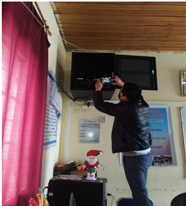
Figura 66. Rack, laboratorio 1, bloque 1.
